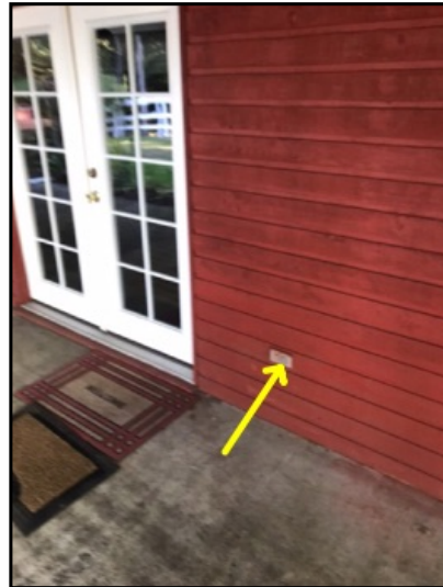
Not GFCI protected.
