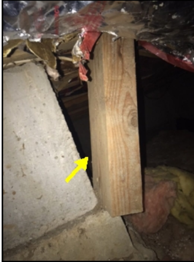
Pier not secured noted.
