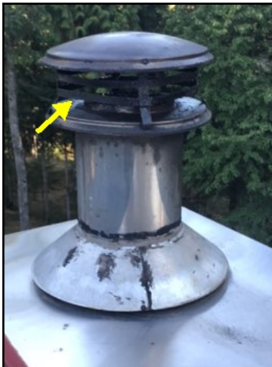
Accumulated creosote noted.
