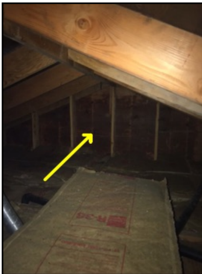
Possible moisture noted.
