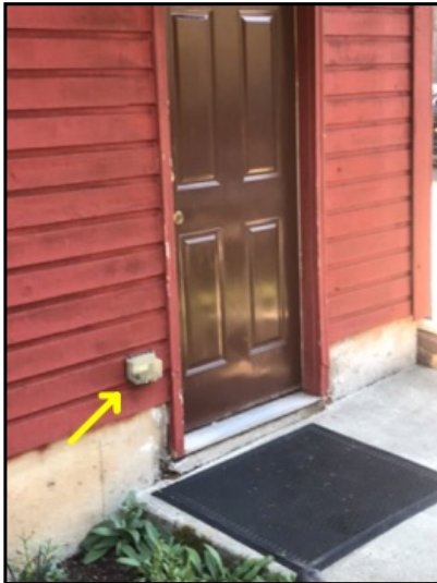
Not GFCI protected.
