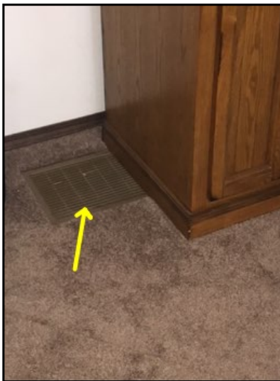
Restricted airflow noted.
